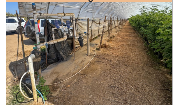
Block-Level Irrigation Controls
